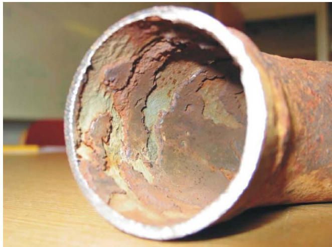
Figure 2: Pipe corrosion caused by carbonic acid
