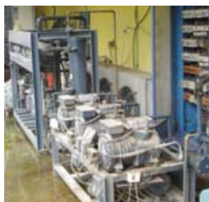
Fig. 1.4 A commercial refrigeration installation using R-22 in a hot climate. This model requires a water spray on the condenser to avoid high pressure and overheating of the compressors. However this causes corrosion and wastes water that is often in short supply. In this case increased electrical hazards are obvious and 'Good Practice' has not been properly considered.
