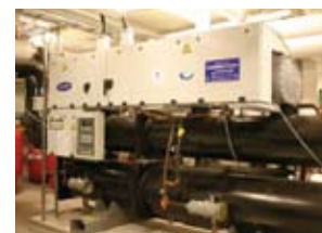
Fig. 2.9 Standard water cooled chiller at an IKEA store in Sweden. The system uses R-134a and is indirect for the evaporator and condenser, minimizing the charge of HFC. It operates as a heat pump in winter and as an air conditioner in summer. To minimize energy consumption, a ground "storage" with drilled holes is used for "free cooling" until the ground temperature increases in late summer when the chiller must start.
