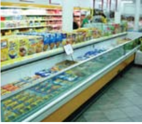
Fig. 2.23 Typical supermarket display cases for a central system with “low temperature” cases in the front and “medium temperature” in the back.
