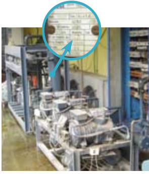
Fig. 1.12 R-22 plant in a warm climate might not have pressure vessels with sufficient design pressure to be used with R-404A. In those cases these vessels should be changed if a retrofit to R-404A is to be done. All pressure vessels should have a plate stating the maximum allowed pressure as shown above.
