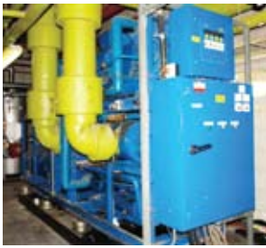
Fig. 2.16 Chiller used for 20 years with R-22 that was retrofitted to R-422D.
