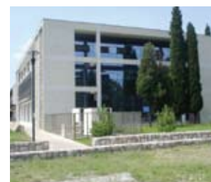
Fig. 2.8 A smaller sized standard air-cooled chiller installation with R-407C installed in 2005 in Montenegro to air condition a public building.
