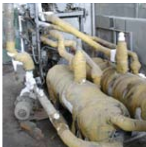
Fig. 2.6 An older model of an air-cooled chiller assembled from "condensing units" used for wine production in Georgia.
