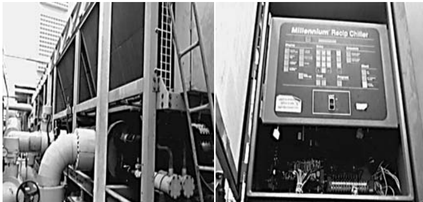
Figures 2 and 3: Far East Square Shopping Complex, Roof Top, Chiller No 3, York Air-Cooled System Model: YDAJ98MU7-50PA
