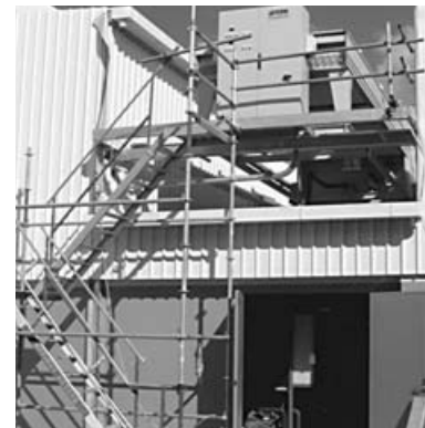
Figure 1: The propylene chiller on the roof and the CO 2 unit in the room under during commissioning
