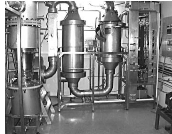
Figure 15: The fluid bed CO 2 heat pump dryer at the NTNU-SINTEF laboratory
