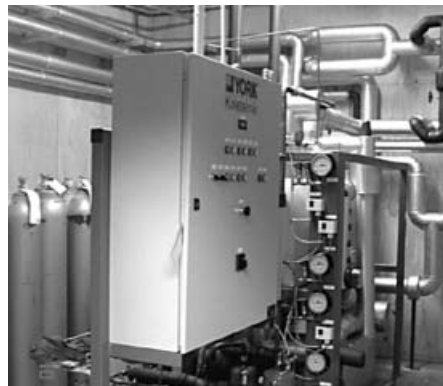
Figure 2: The CO 2 part of the plant and some of the CO 2 cylinders in the background
