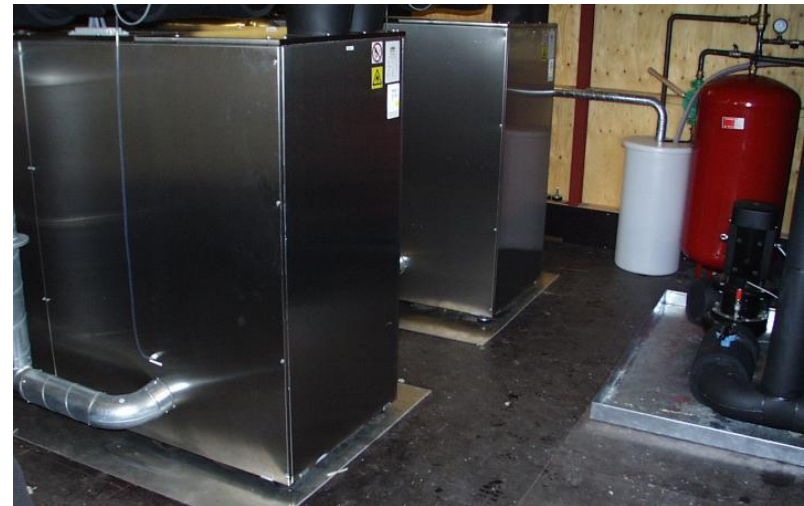
Two indoor Hydro-Carbon chillers
