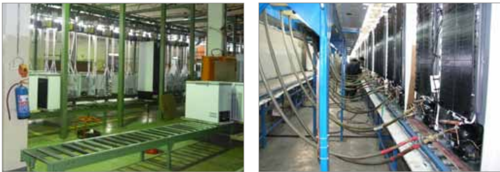
Figure 15: On-site evacuation line
