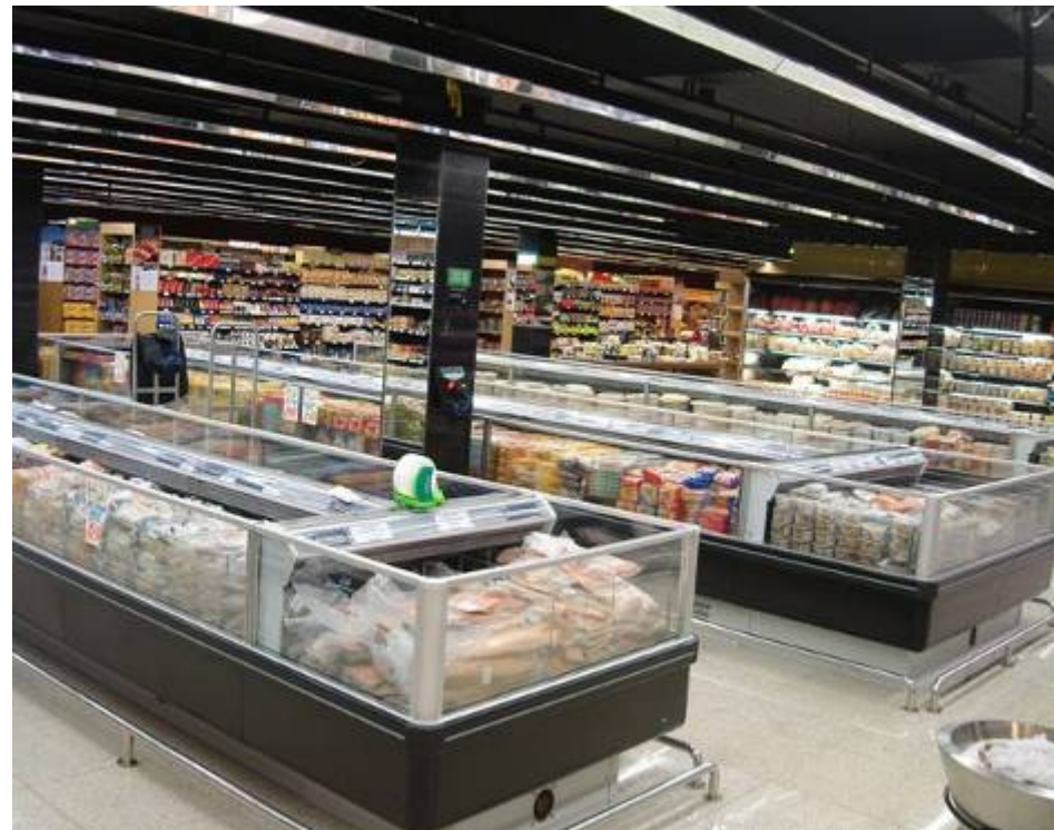
The frozen products section of the new store: Low temperature islands with CO 2
